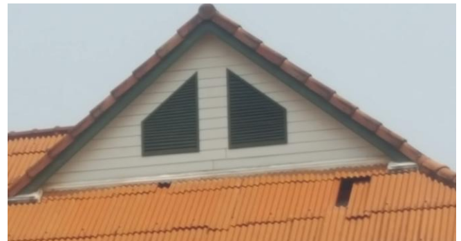
Breakage of the roof tiles
